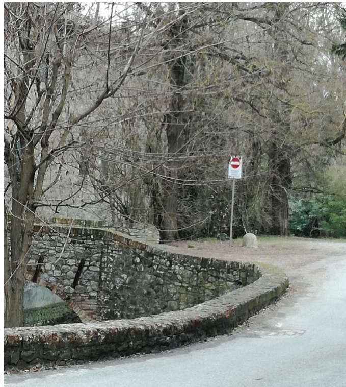
Figure 6. 16 LOII reported that the stream banks and part of the street on the right are made by the debris of the old shed of a farmer living there, who had pulled down it and dropped it into the stream
