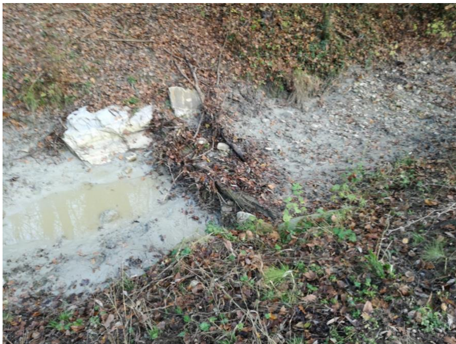
Figure 6. 23 One of the interventions: leaky dams with tree roots in the Rio Bianello to slow down the flow
