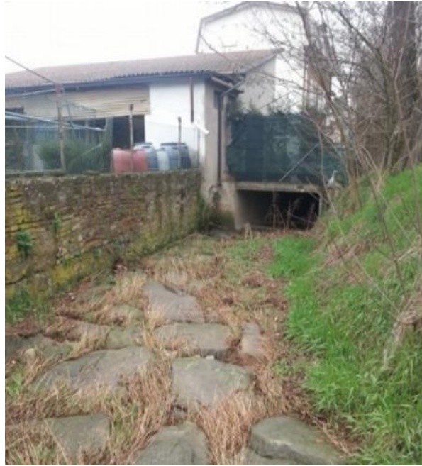
Figure 6. 21 The Rio Montefalcone channeled and culverted in the middle of Bibbiano town (source LIFE RII)
