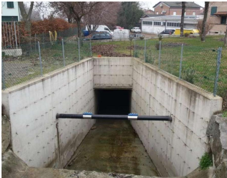
Figure 5. 7 The Rio Enzola flows culverted in Bibbiano town
