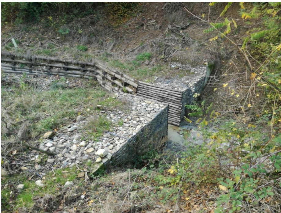
Figure 6. 25 One of the works: an enlargement (on the left) and then a narrowing (on the right) of the stream bed to provide flooding areas upstream for slowing down the flow
