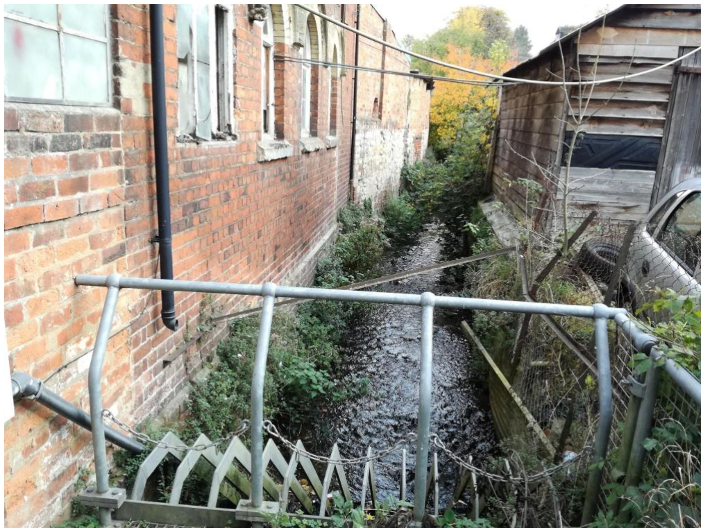
Figure 5. 6 The Slad brook flowing behind the houses downstream. Here the culvert begins. The grid has been put here after the 2007 flood to avoid blockage causing flooding (see next paragraph)
