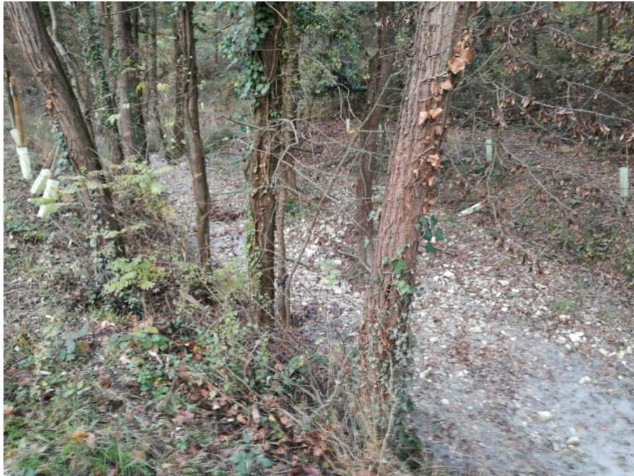
Figure 6. 24 One of the works: enlarging the stream bed and keeping trees in it to reduce the water speed
