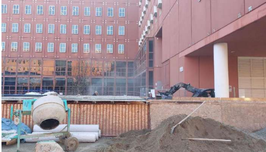
Figure 3.17. Overview of part of the square during the removal of materials, where dust resuspension becomes clearly visible.
