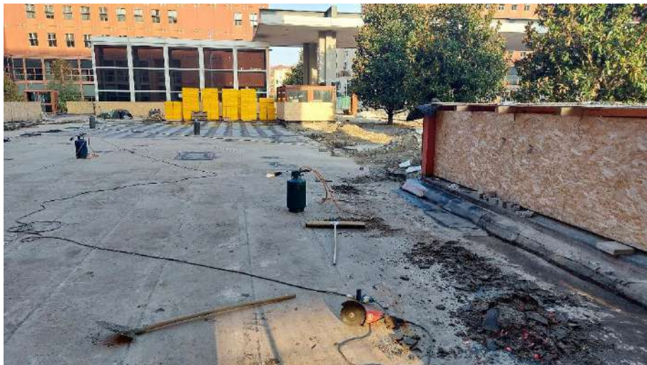
Figure 3.16. Overview of part of the square during the positioning of the insulating material.
