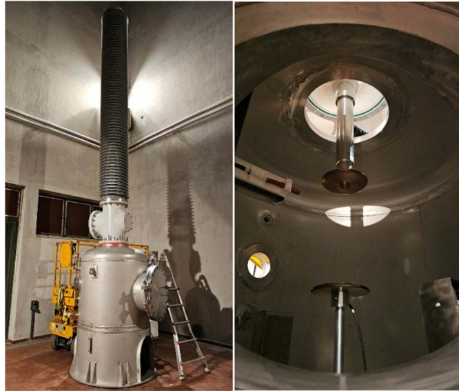
Figure 9. Picture of the external (left) and internal (right) view of the new experimental device for HVDC-GIS testing.
