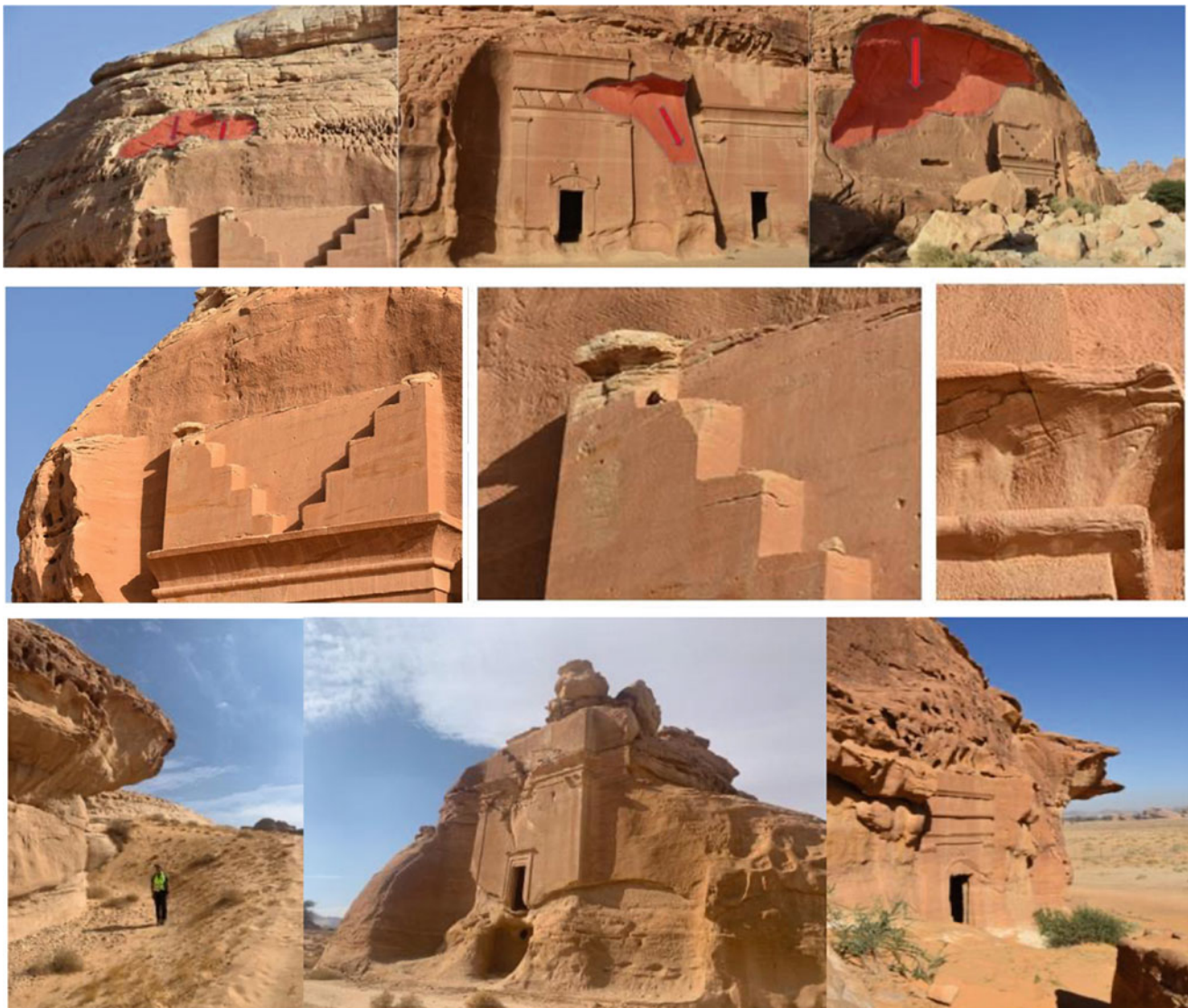
Fig. 10 Example of the main instability processes affecting the different tombs in Hegra: upper sequence of photos stands for rock slide and free fall; middle sequence is reporting small cracks, fractures and
