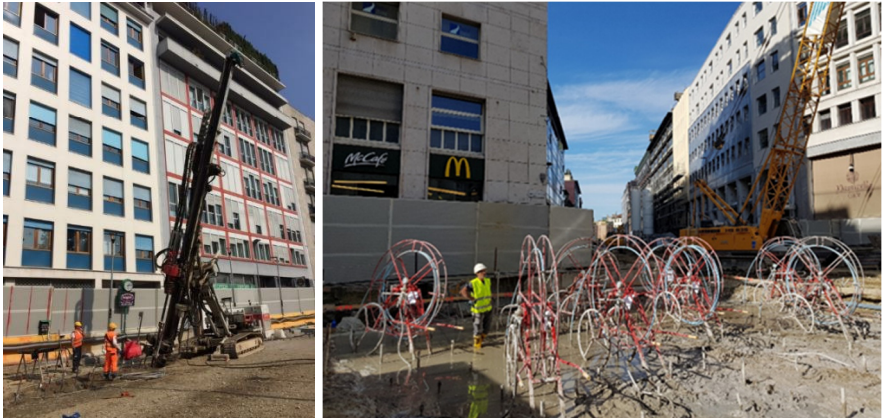
Figure 4: drilling and grouting works, respectively on the left and on the right. (Pettinaroli A. et al., 2019)
