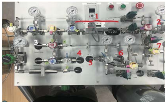
Figure 4: Gas handling system
