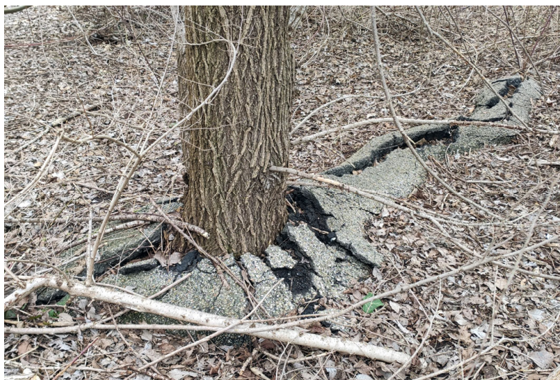
Figure 14. Ulmus spp. root action in the fragmentation of the asphalt surface (“natural desealing”).
