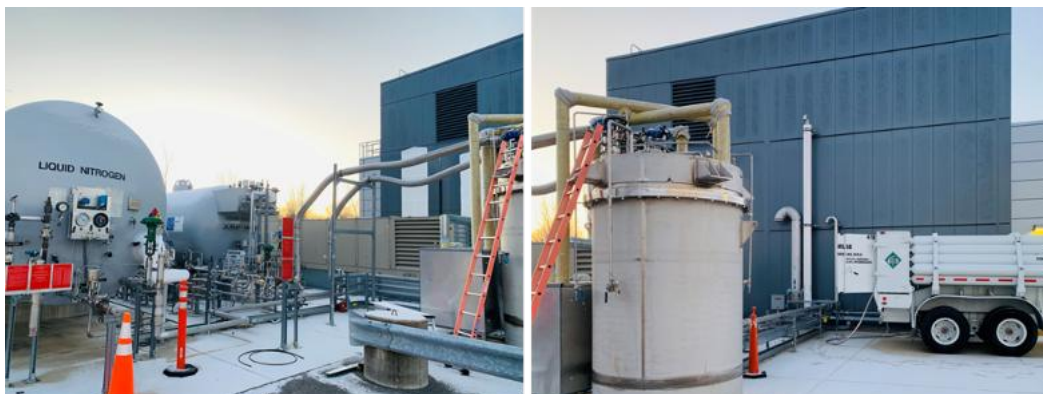
Figure 6. Cryogenic dewars and fill filter.
