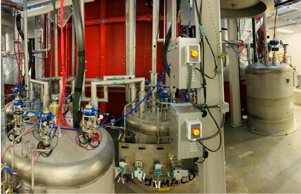
Figure 12. Three LN 2 pump boxes (left) and West LAr pump box (right).
