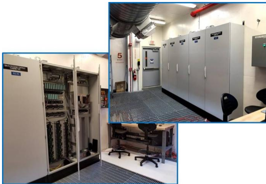
Figure 53. Cryogenic control cabinets.
