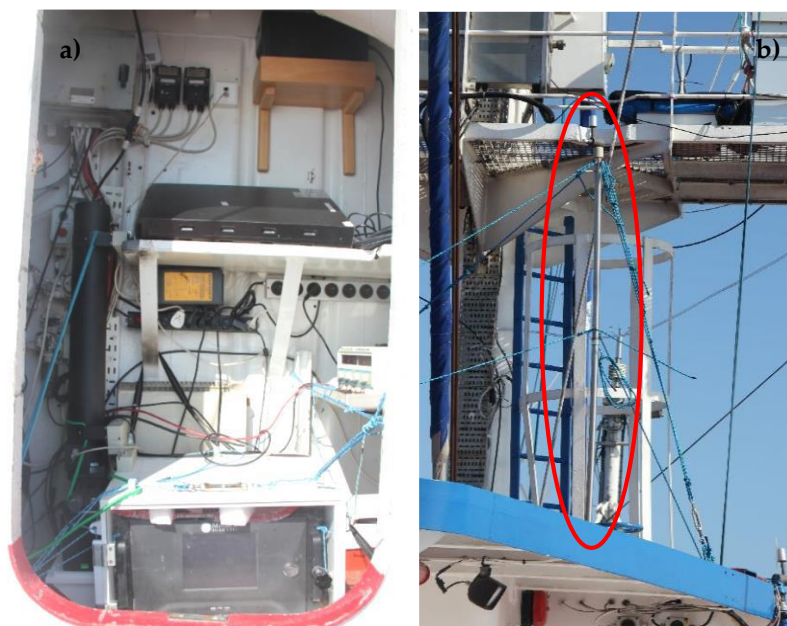
Figure 13. Aethalometer inside a special built recovery box in the sealed room (a). metal hollow containing the sampling line and ending with a \text{PM}_{2.5} cyclone (b).
