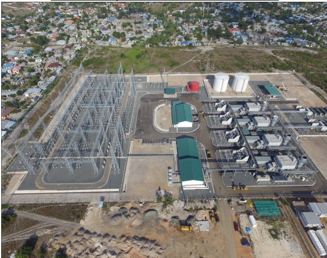
Picture 8.1: Kinyerezi I Power Plant in Dar-es-Salaam
