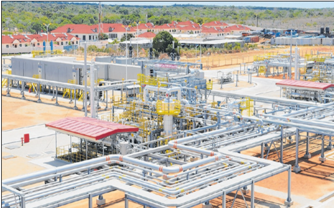
Picture 6.2: Madimba Power Plant in Mtwara
