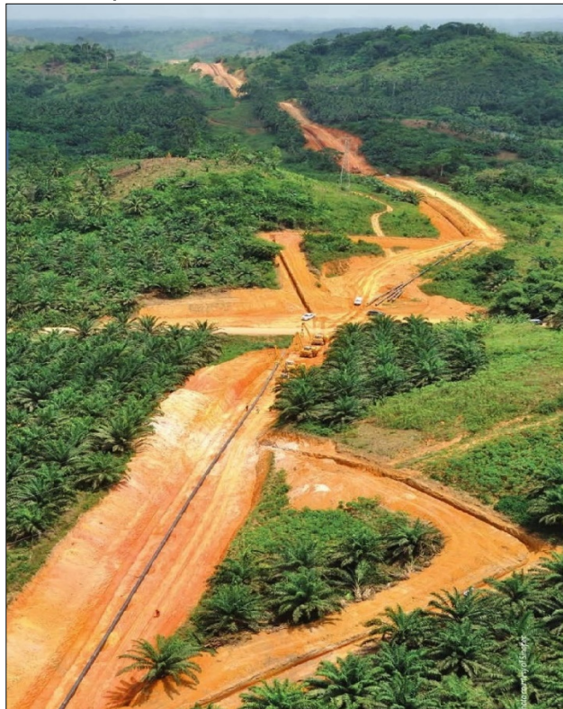
Picture 5.4: Pipeline from Atuabo Gas Plant to Aboadze
