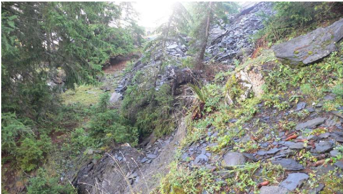
Figure 40 – stepped appearance at right-flank of the rockslide
